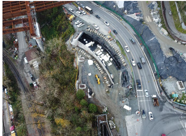
Figure 4: Aerial view of the ongoing construction in New Westminster, including the new exit ramp that will provide a direct connection from the new bridge to E. Columbia Street.
