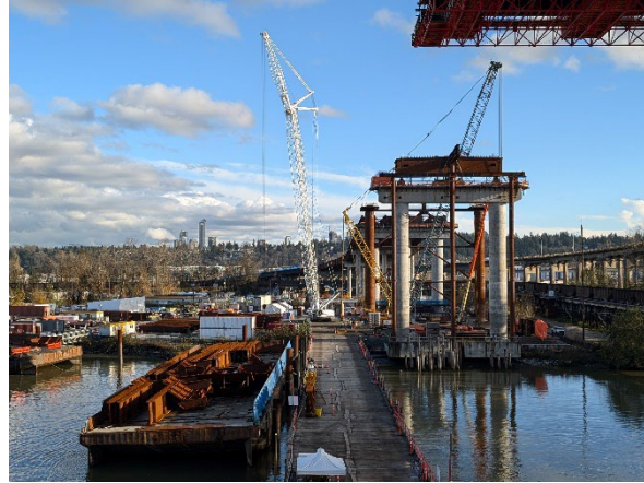
Figure 2: In Surrey, end span girder erection is progressing steadily, with steel girders stored on the barge in the foreground, ready to use.
