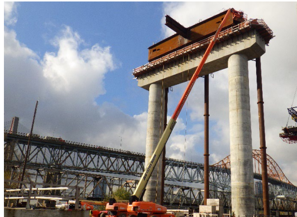
Figure 4: Steel crossbeams were installed on top of pier S2 as part of the girder installation for the end span.
