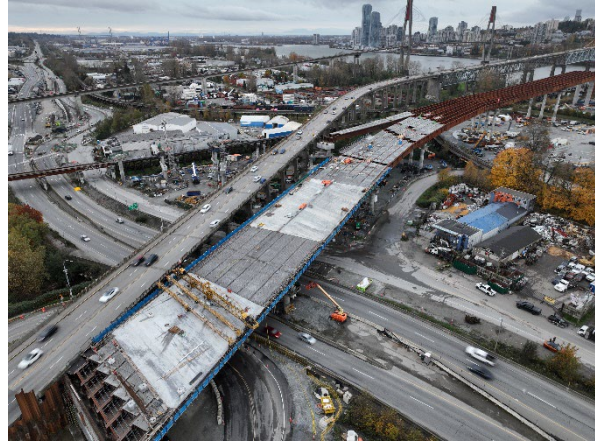
Figure 2: In Surrey, concrete decks were poured to create a smooth surface before asphalt paving.
