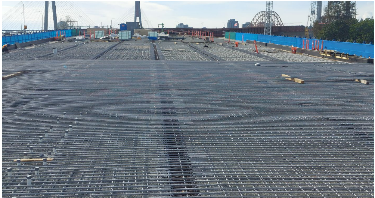
Figure 4 – In Surrey, crews are installing rebar over the precast deck panels and preparing for the first concrete deck pour on the South Approach.
