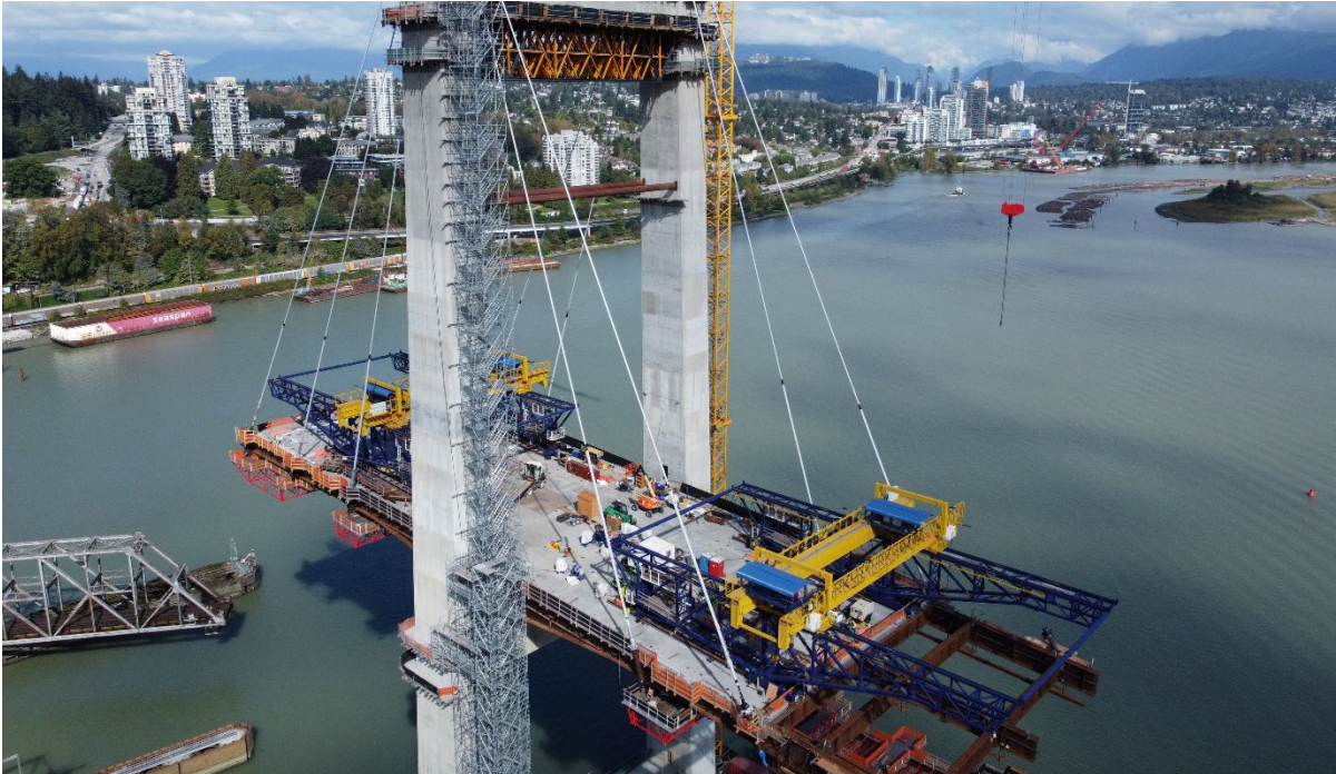
Figure 2 – Girder erection, deck panel, and stay cable installation for main bridge continues.
