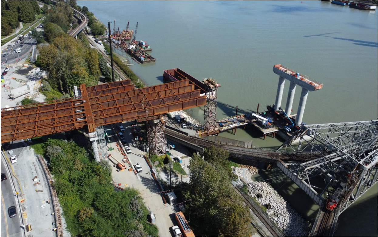
Figure 3 –In New Westminster, girders are installed above Front Street and extend towards the temporary support tower.
