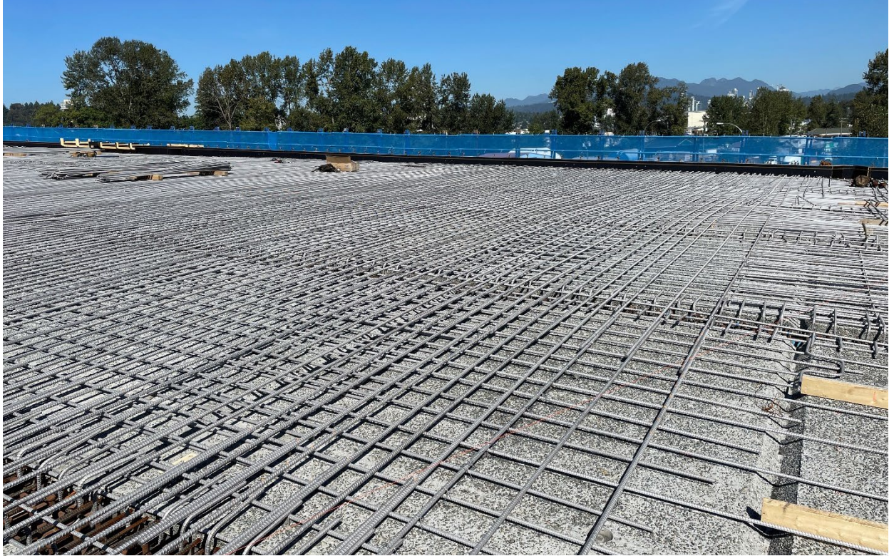
Figure 3 – In Surrey, crews are installing rebar over the precast deck panels on the south approach.
