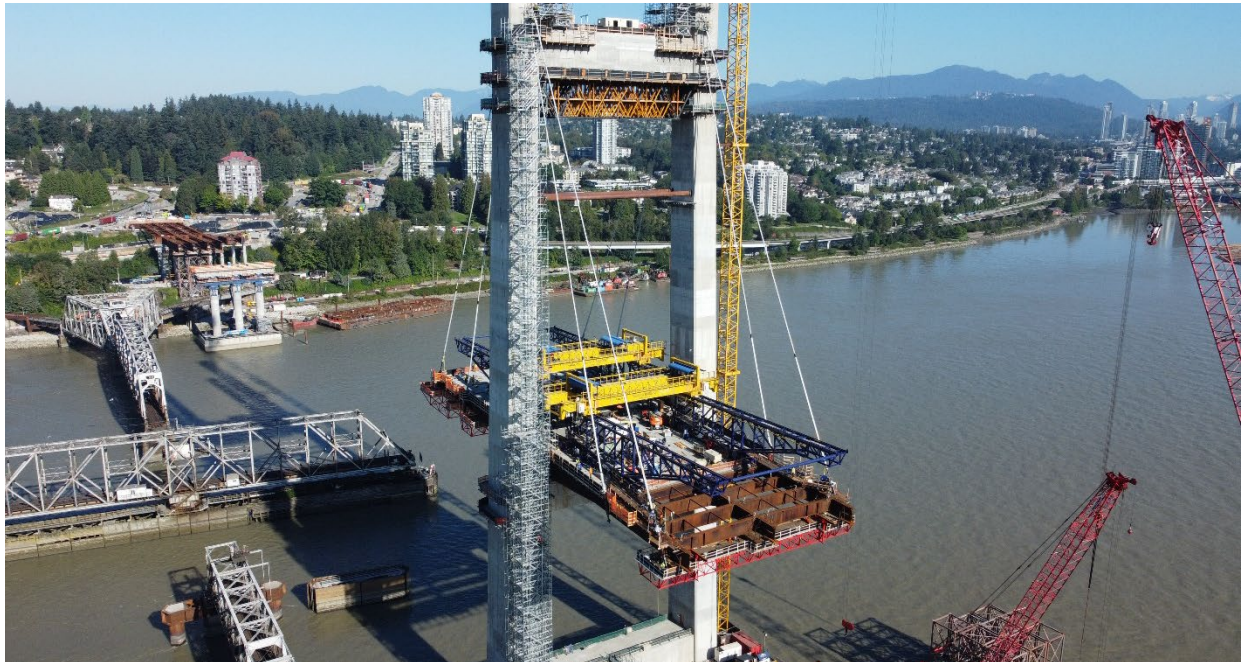
Figure 4 – Girder erection, deck panel, and stay cable installation for main bridge continues.
