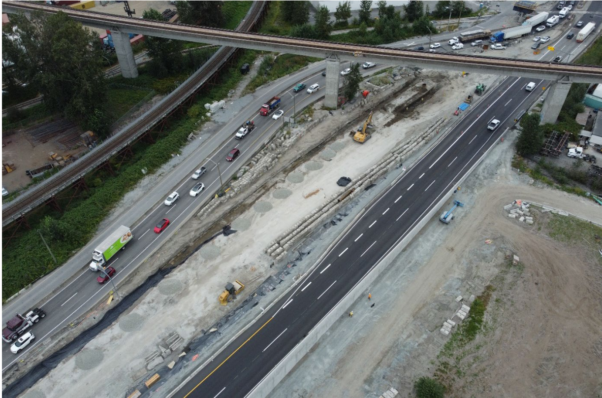
Figure 1 – In Surrey, crews started to construct the westbound portion of the Old Yale Road Overpass.
