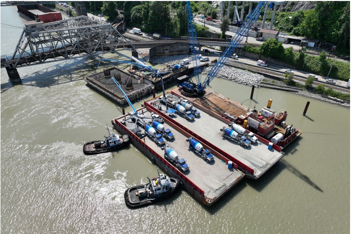
A fleet of concrete trucks completing a large concrete pour for the pier near the New Westminster shoreline.
