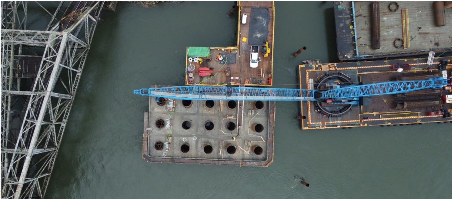
Overhead view of rebar being installed at the in-river foundation near the New Westminster shoreline.
