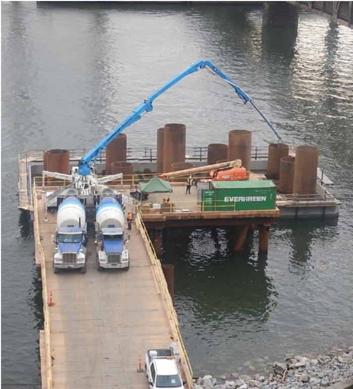
Piles being filled with concrete for the in-river foundation near the New Westminster shoreline.
