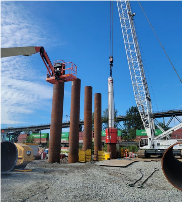
A hydraulic hammering machine driving steel piles as part of foundation construction in Surrey.
