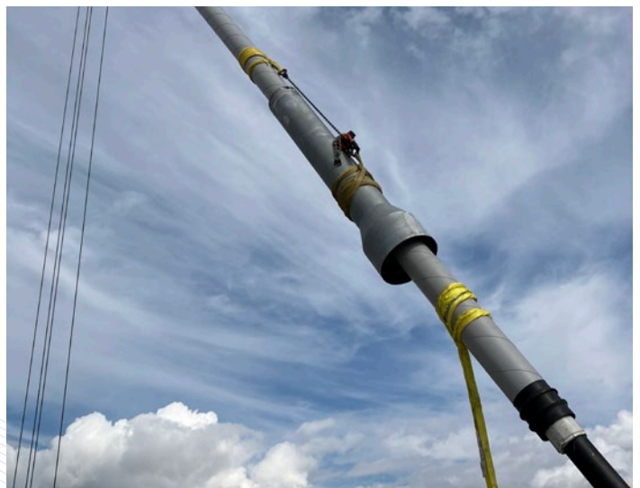
Cables and cable tube at the base of the stay cable.
