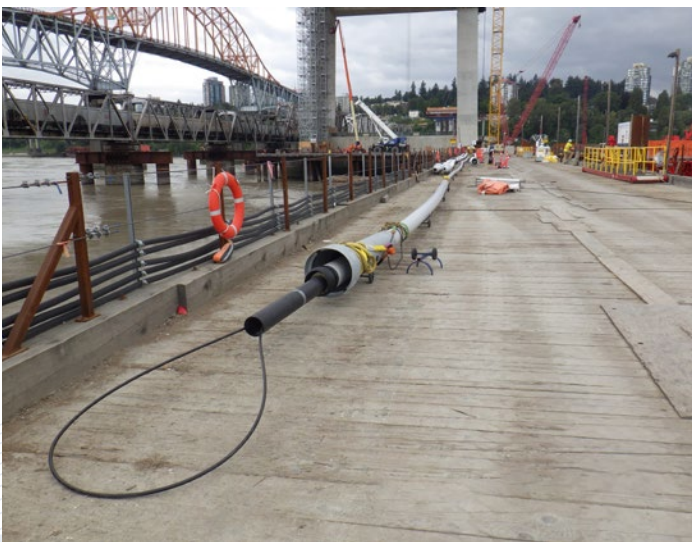
A stay cable tube at base of the bridge tower is ready for installation.
