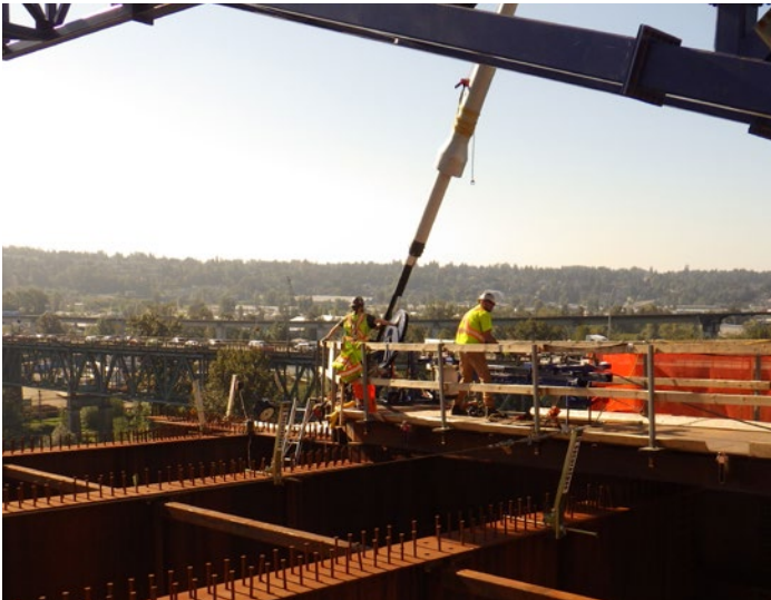
Crews on the bridge deck install cable strands in the stay cable tube.
