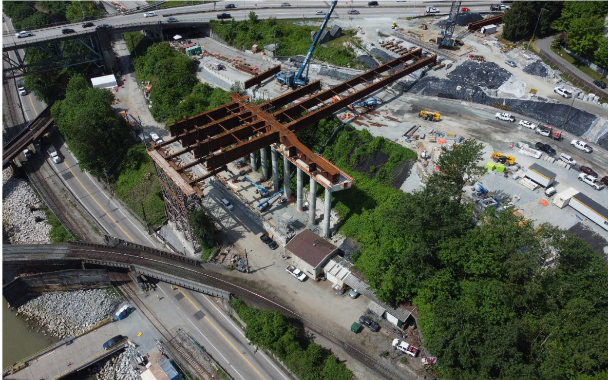
Figure 3 – Aerial of the north approach girder installation from over Columbia Street in New Westminster.
