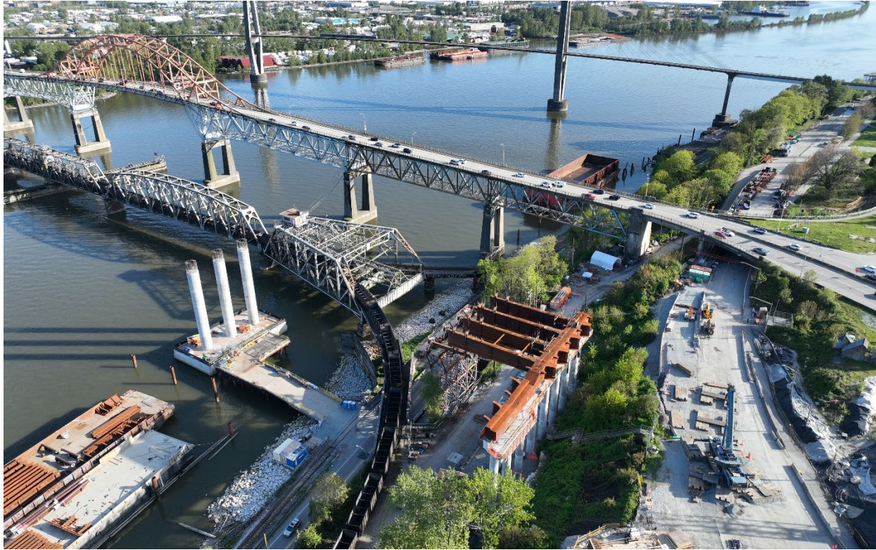
Figure 3 – Aerial of pier N2 in New Westminster girder installation from N2 to the temporary support tower.
