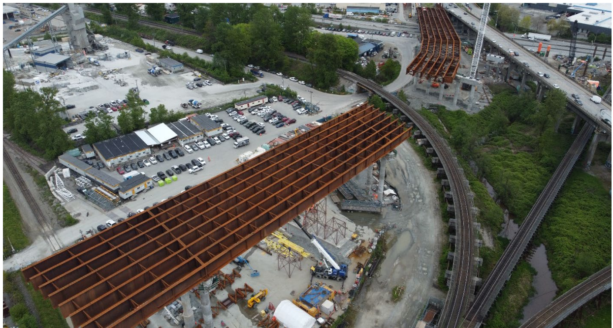
Figure 4 – Aerial of girder installation between piers S4 to S5 and S6 and the South Abutment.
