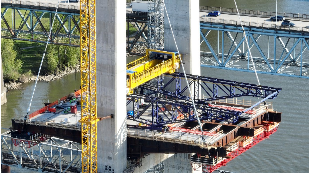
Figure 2 – Crews installed the first pairs of cable stays on either side of the bridge tower.
